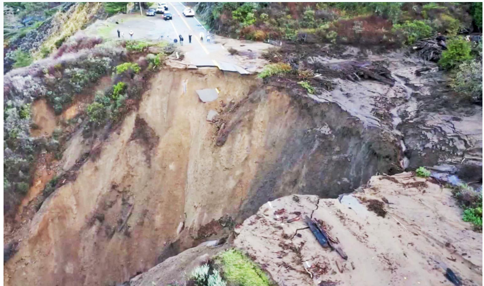
Highway 1 North of Big Creek Bridge wash out
