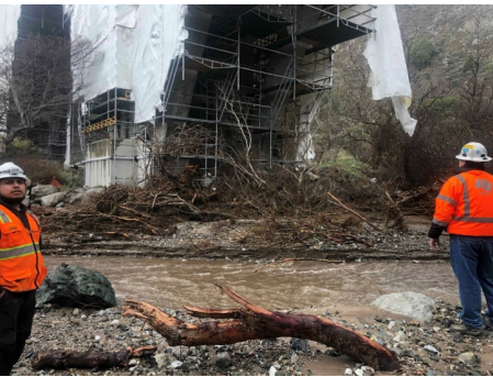
Flooding and debris
