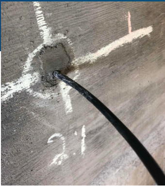
Cathode wire connection to the reinforcing steel
