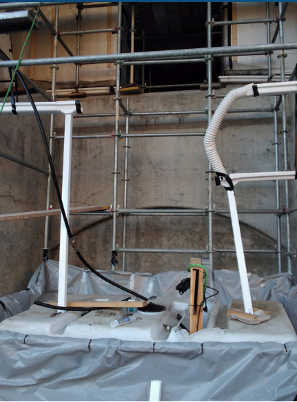
Collection tank placed at the bottom of each pier to capture waste water for recirculation
