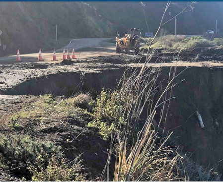
Highway 1 South of Big Creek Bridge erosion
