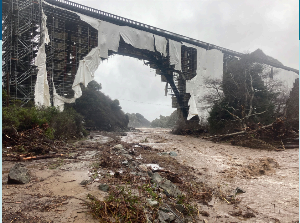
Aftermath of heavy winds and flooding
